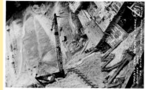
Twenty Ton Capacity Crane, Boulder Da
