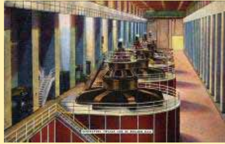
25366N Generators, Nevada Side of Boul
